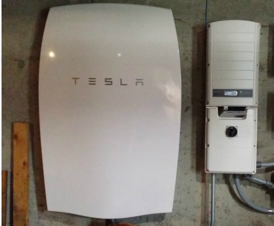
(a) Tesla Powerwall
